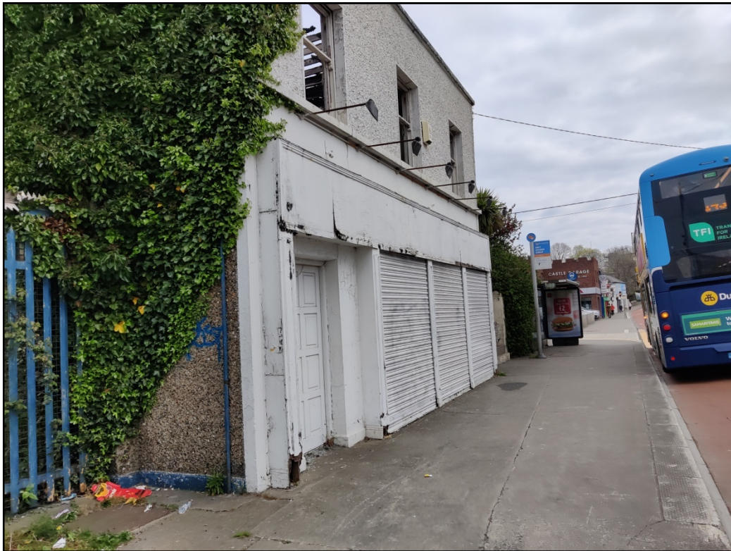
Plate 8 View of former shop and dwelling building (II) fronting Castle Street, looking E.
