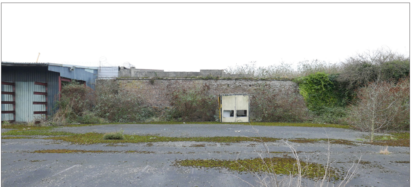
Brick wall near the north west corner of the site. This appears to be the partial remains of a wall that once bounded a walled garden. It is proposed to retain, repair and refurbish this wall
