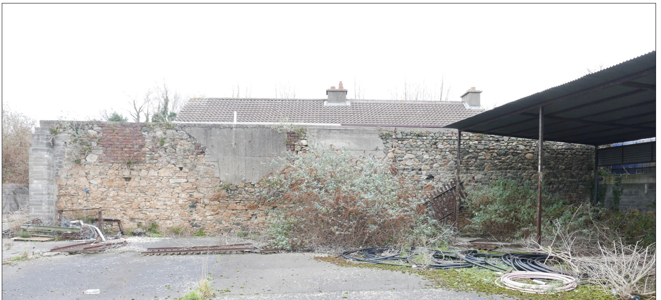
Rear boundary wall of Nos 15 and 16 Dwyer Park. It appears to be fragments of the walls of small buildings in the course of the construction of Dwyer Park. It is proposed to replace it with a more stable wall
